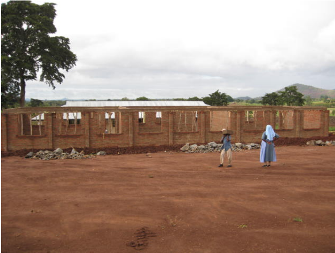
Construction continues with the Form II block at Usambara Girls School in Tanzania
